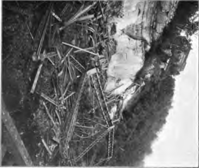
FIG. 1.—SMITH AVE. VIADUCT. VIEW LOOKING NORTHEAST SHOWING PARTS OF SHORE TOWER, 170-Ft. SHORE SPANS AND TWO 60-Ft. PLATE GIRDERS.
